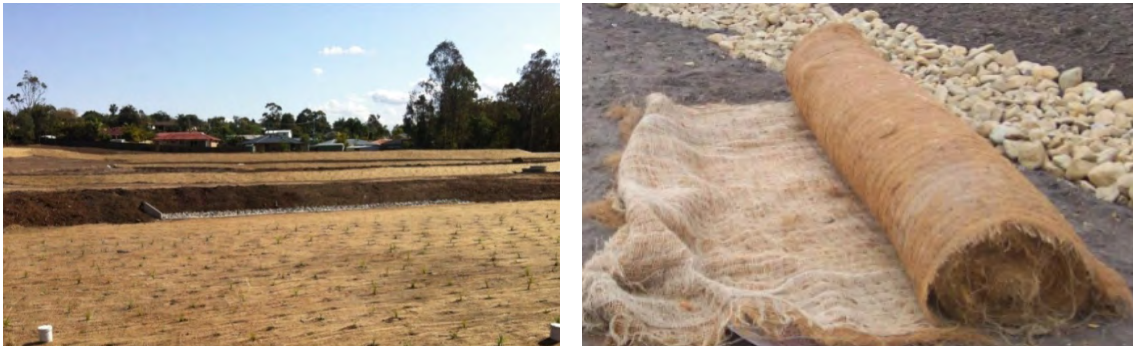
Figure 2.14 Jute netting in a bioretention system.
