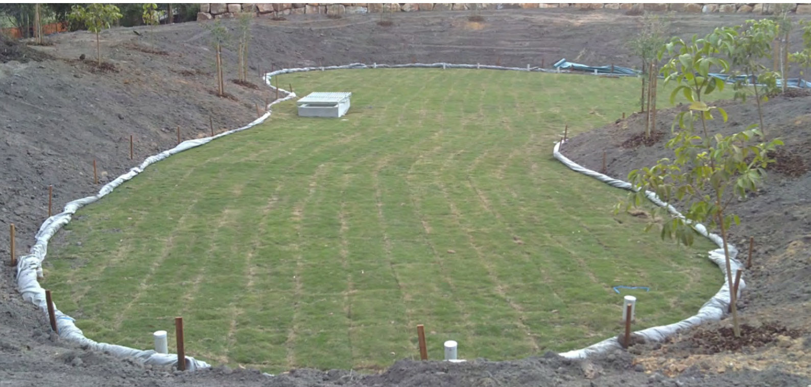
Figure 2.33 Use of temporary measures to protect a bioretention system during the building phase.
