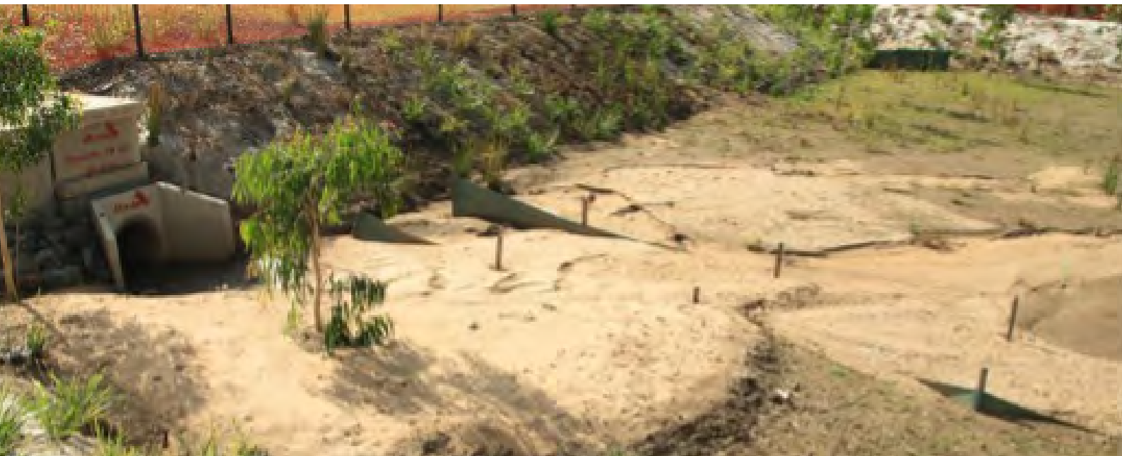
Figure 2.21 Sediment from building phase activities in a bioretention system.
