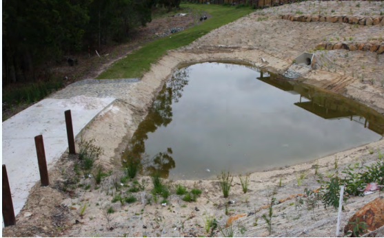
Figure 2.27 Use of a bioretention system as a HES basin during the building phase.
