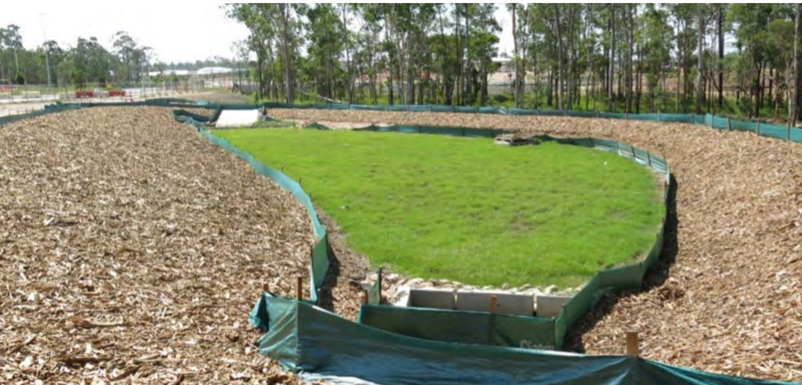
Figure 2.24 Use of temporary measures to protect a bioretention system during the building phase.
