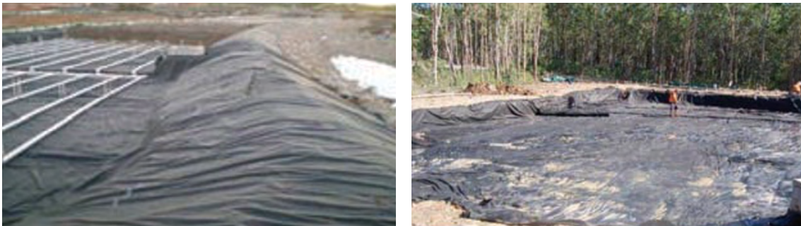
Figure 2.3 Filter cloth liner in a bioretention system.
