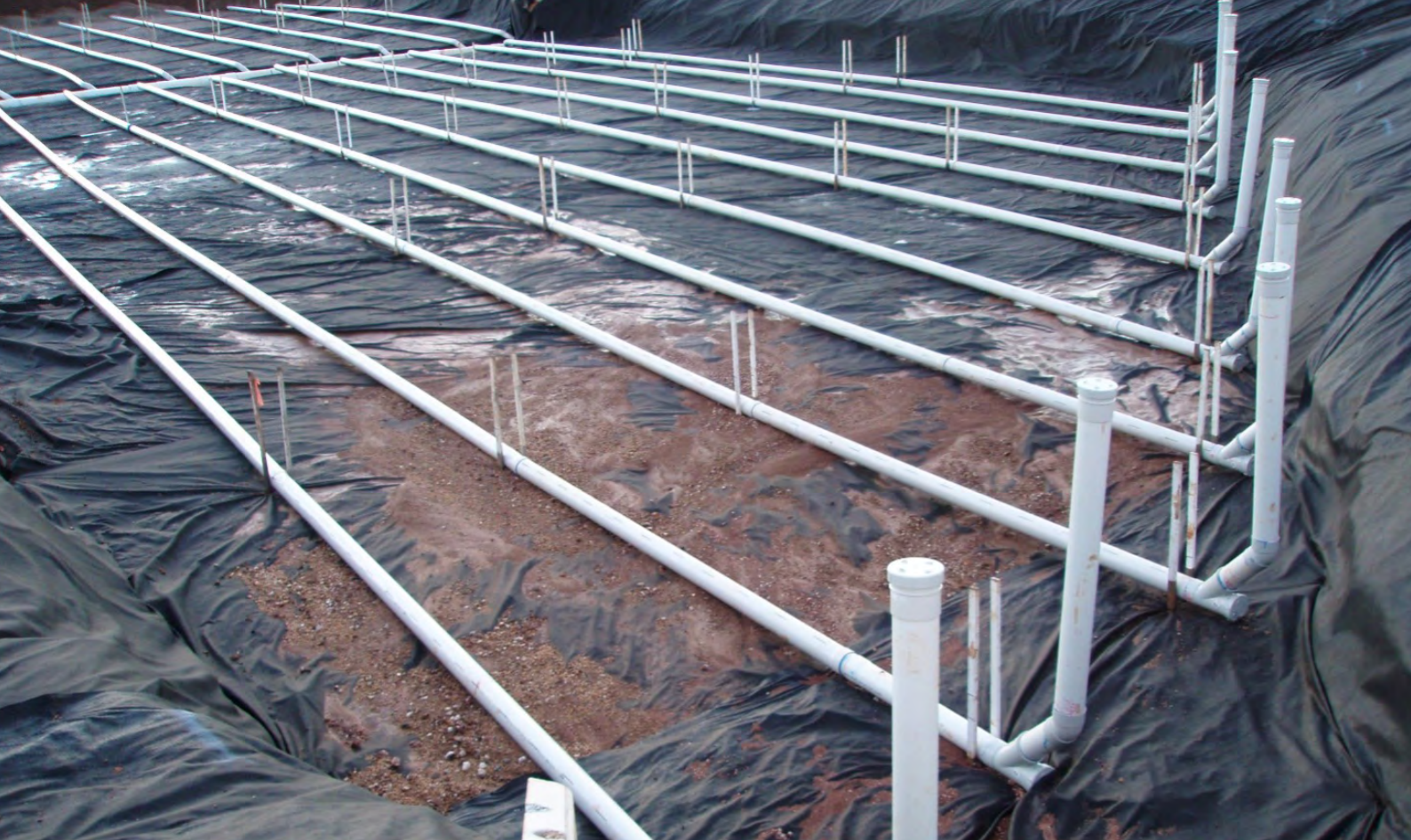
Figure 2.30 Cleanouts in a bioretention system.
