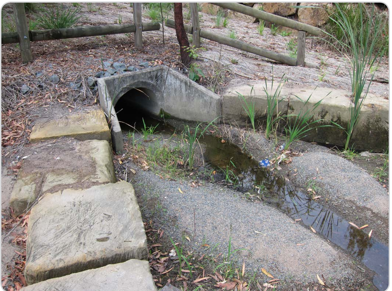
Figure 43: Coarse sediment from upstream building sites in the coarse sediment forebay
