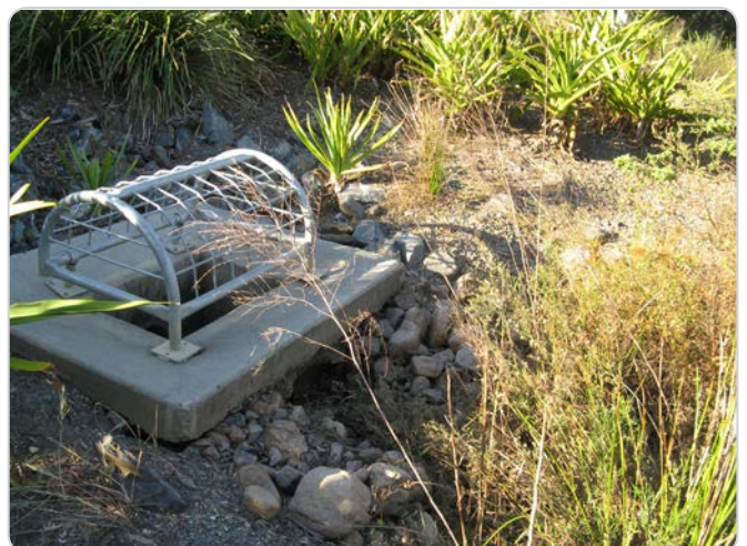
Figure 21: A System With a Scour Hole
