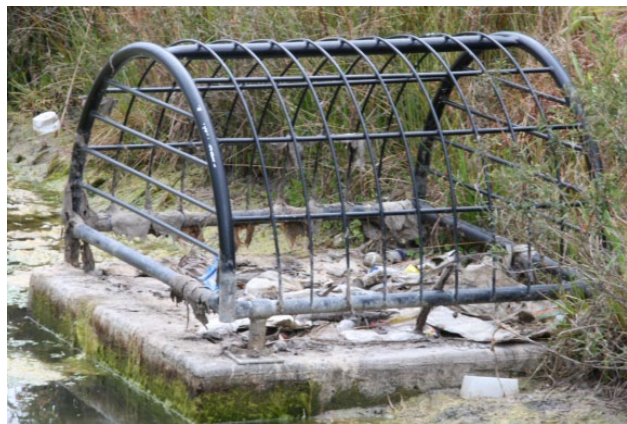
Figure 16 Litter blocking outlet pits
