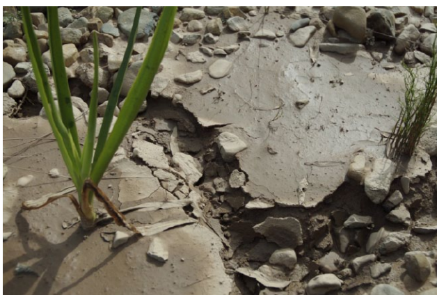
Figure 18 Examples of a bioretention surface that has been blinded with clay-like sediment deposition
