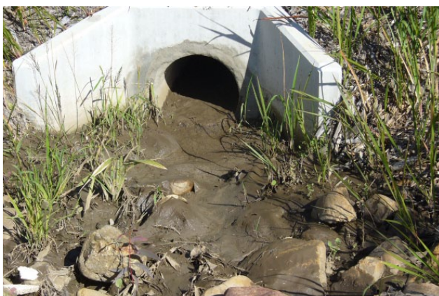
Figure 17 Sediment accumulated at an inlet
