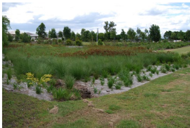
Figure 14 Erosion at the transition between a swale and bioretention system causing ripping of the jute mat
