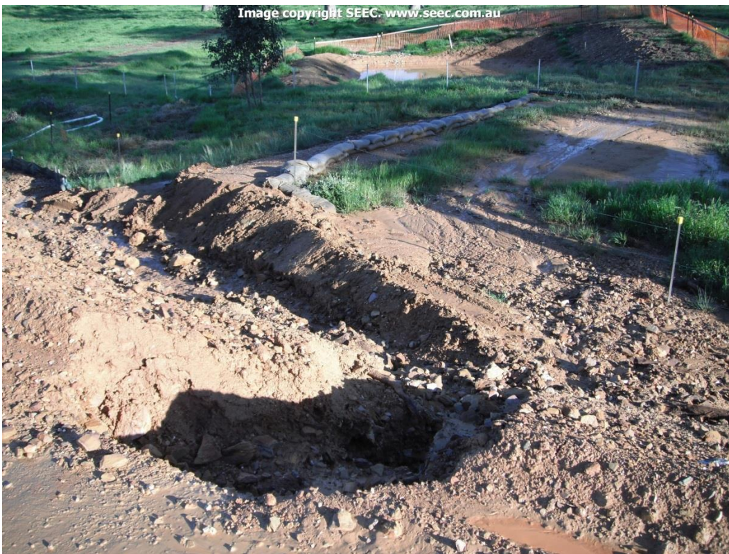
Figure 3 The scour extended down the batter and created a channel which diverted dirty water away from the sandbag-lined berm which should have taken dirty water to the sediment basin (visible in the distance). As a result, dirty water missed the basin and flowed directly offsite.
