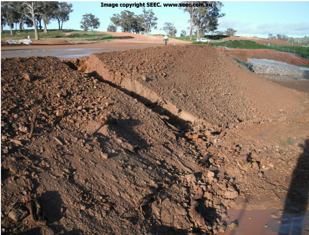
Figure 2 Scour of the fill embankment caused by lack of drainage control. Lined batter chutes as shown on the ESCP (Figure 1) had not been installed prior to rainfall.
