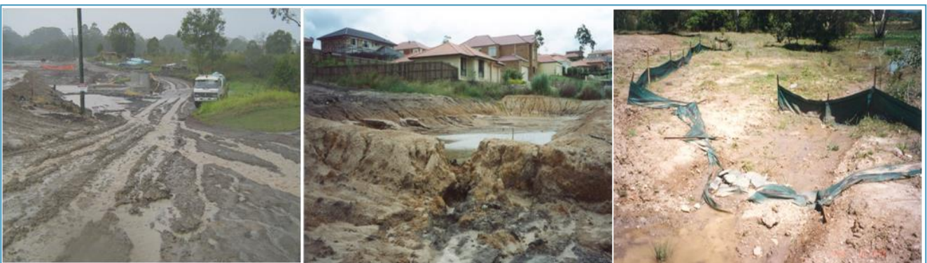
Figure 5 Examples of on-site impacts due to poor erosion and sediment control
