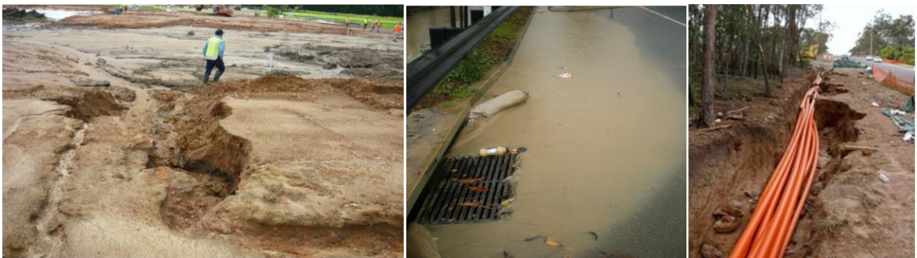
Figure 6 Erosion and sediment loss due to poor on-site ESC management
