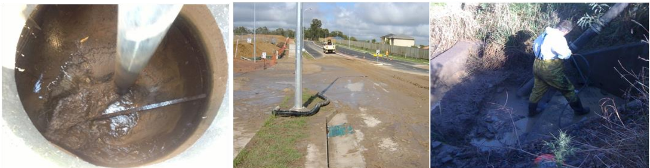
Figure 8 Sediment accumulated within Council infrastructure
