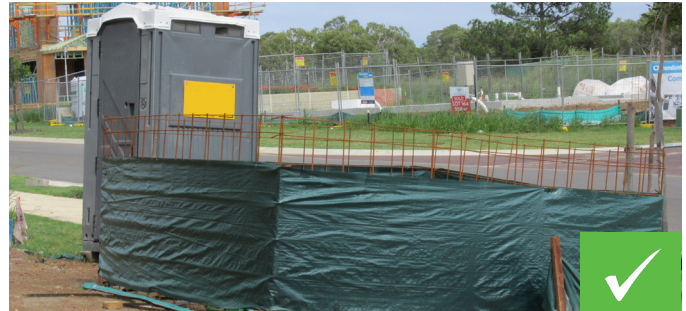
Typical fabric wrapped mesh cage. (Source: Healthy Land and Water)
