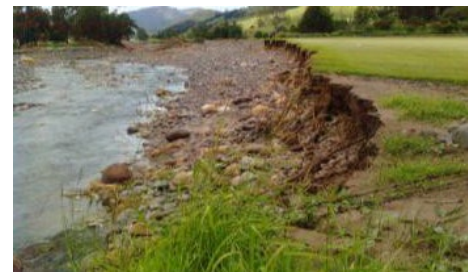
The depth, duration and velocity of flow as well as the erodibility of the bank and floodplain material will influence the severity of bank erosion.
