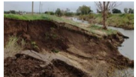
Mass failure, or slumping, occurs when chunks of the bank slide or fall into the stream, often leaving near vertical banks.
