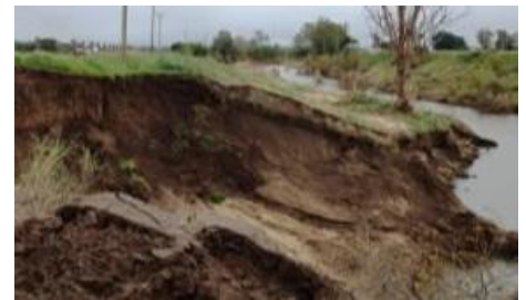
Mass failure, or slumping, occurs when chunks of the bank slide or fall into the stream, often leaving near vertical banks.
