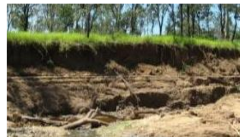
Bank scour occurs due to the action of flowing water removing soil from streambanks. Bare or poorly vegetated areas are especially prone.
