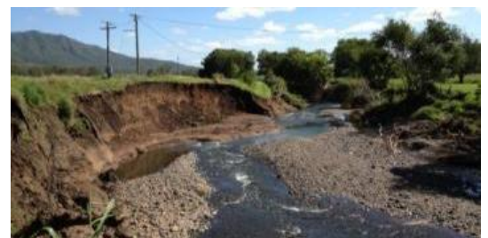
THORNTON: Both mass failure and erosion scour has occurred in the example above resulting in a loss of land and the need to relocate farm tracks and power infrastructure.
