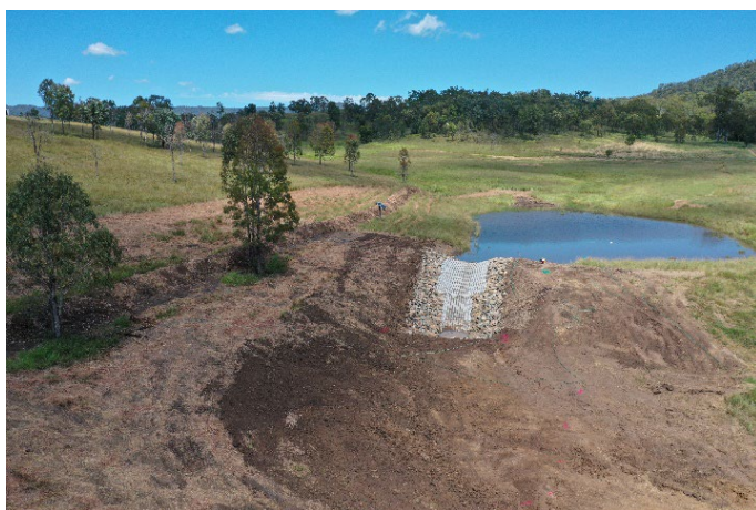
Figure 8. After construction the bare areas were seeded with a mix of productive perennial grasses and a cover crop.
