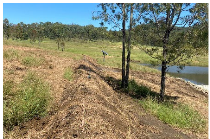
Figure 9. A contour bank was installed to divert runoff away from the restoration site.
