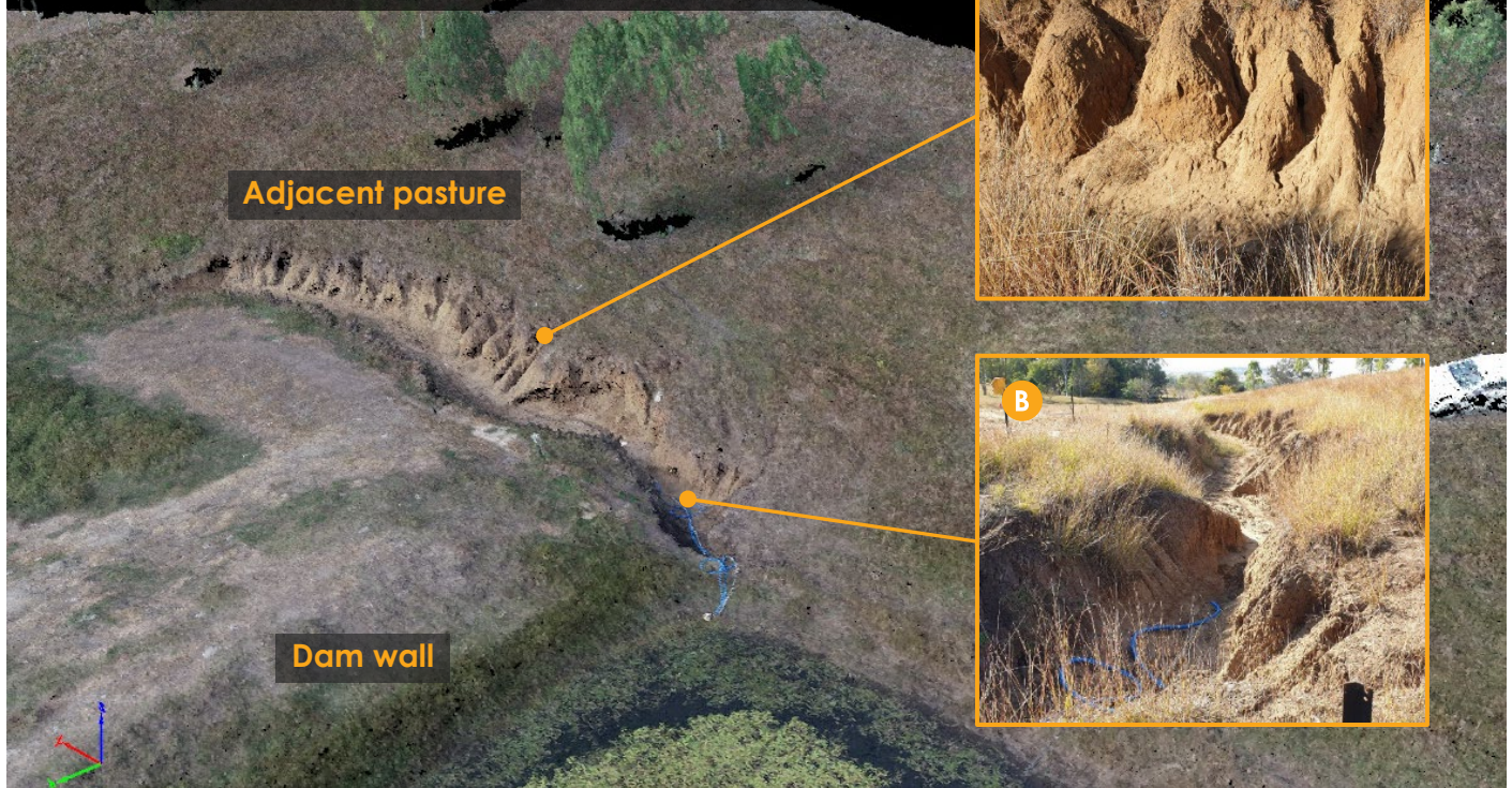
Figure 2. Aerial view of the erosion site before the erosion control work began. Inset A shows where runoff from the adjacent pasture was causing further damage. Inset B shows where the gully erosion continued from the dam wall down into the paddock.
