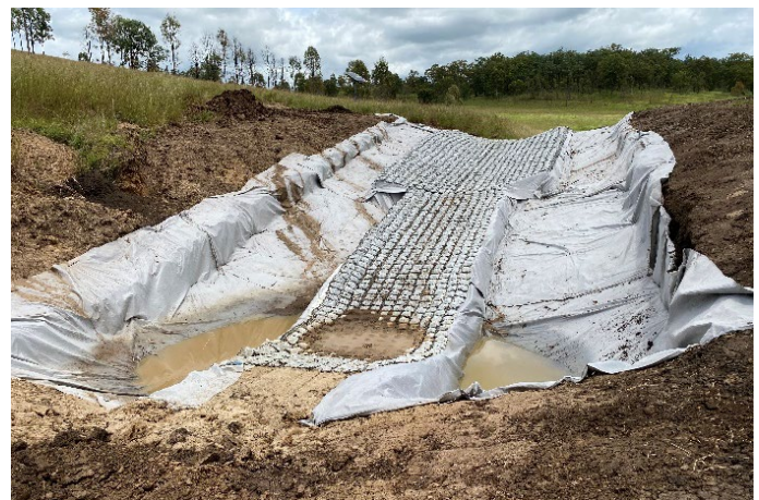
Figure 7. Geofabric overlayed across the entire chute and trenching and cement matting overlayed across the chute.
