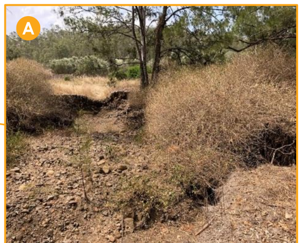
Figure 2. Aerial view of the erosion site before the erosion control work began. Inset A shows the erosion site looking upstream.
