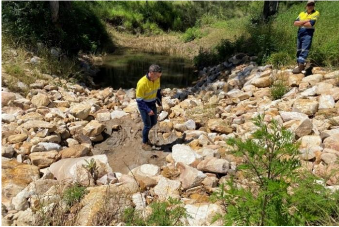
Figure 8. Some of the rock had been displaced during a rainfall event exposing the underlying damaged geofabric and soil.
