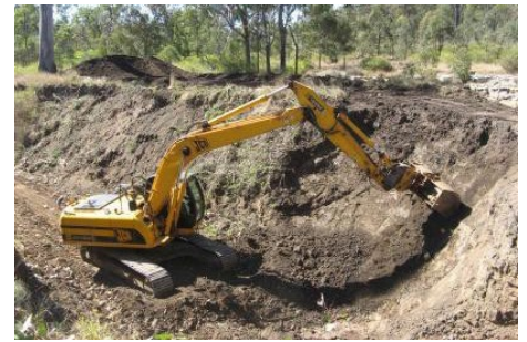
Battering the banks of the gully reduces mass failure and provides a platform for vegetation to establish to protect the soil.
