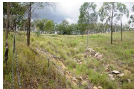
Topsoil spread over the rock chute aided the establishment of grasses that help hold the structure in place. It survived the 2011 and 2013 flood events.
