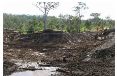
Constructing the control dam across the dual gully heads included compacting the soil to improve the structural integrity of the dam.
