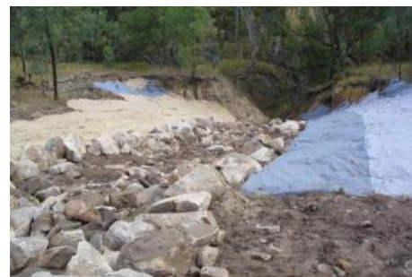
A rock chute was designed for the catchment size with an erosion control blanket built into the design.
