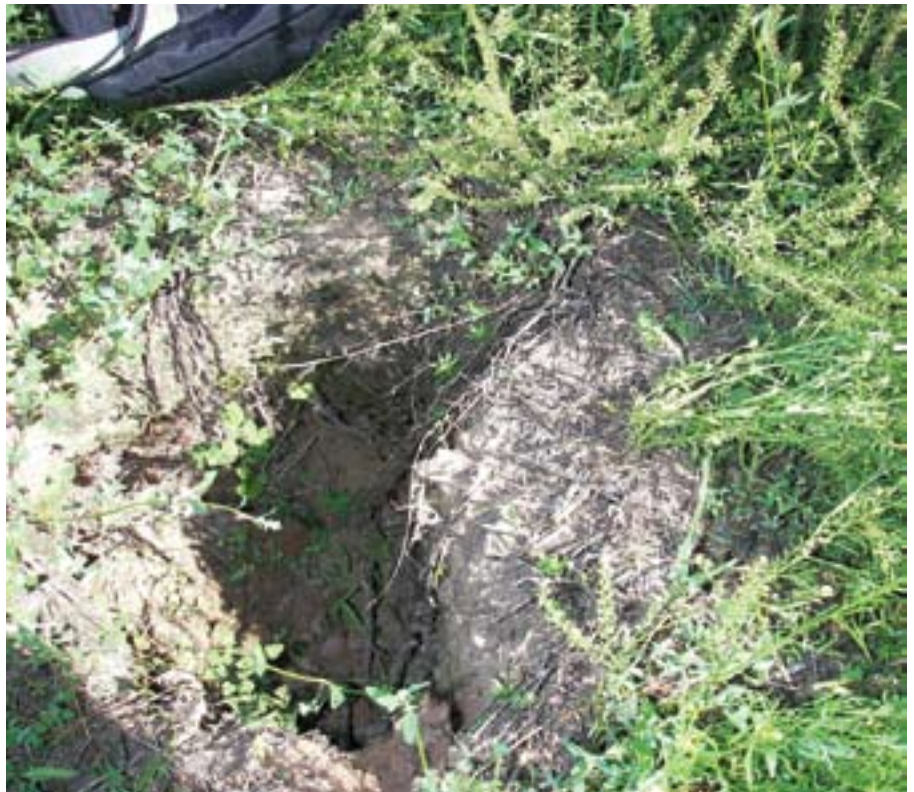
Lethal hole: Tunnelling is common in a number of areas of the Lockyer and nearby Marburg and Bremer catchments. Subsoil dissolves and is washed away, causing the surface to collapse, forming gullies. These sediments can stay in suspension reaching waterways.
