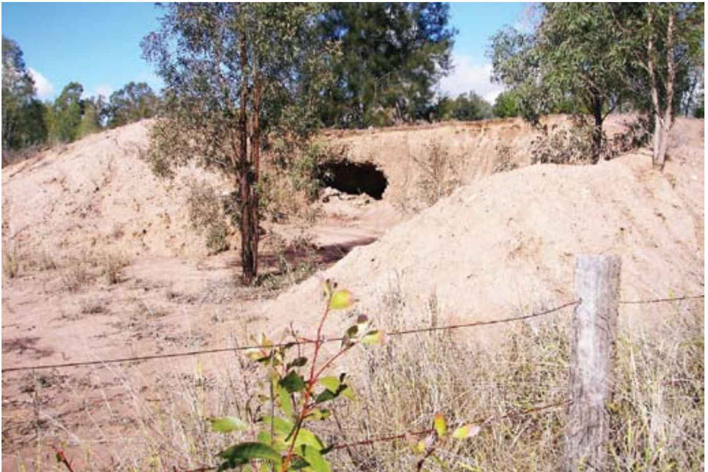
A broken dam in the Withcott area on the highly erodible soils typical of the Marburg geological formation. Construction of dams in this soil need particular attention to compaction and other preventative measures.
