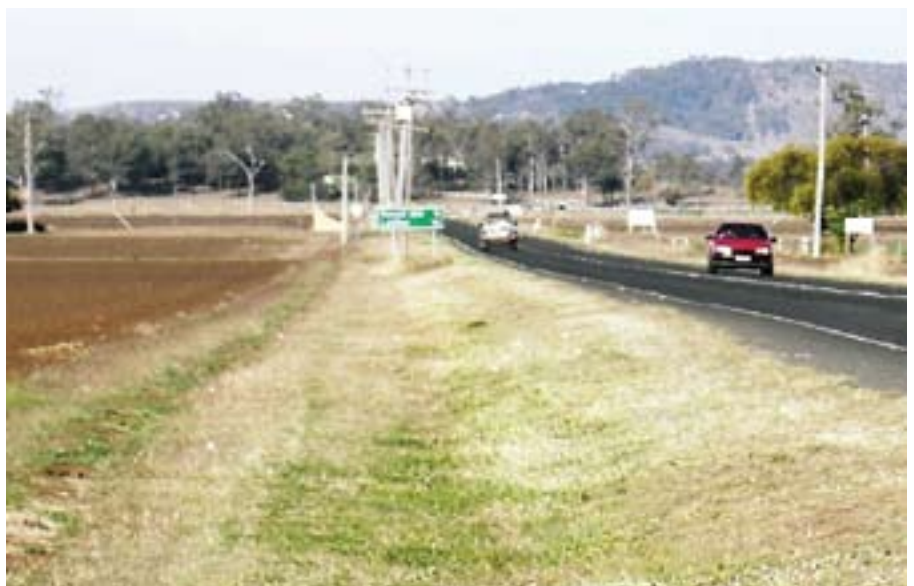
A well grassed roadside table drain reduces erosion in high flow periods.
