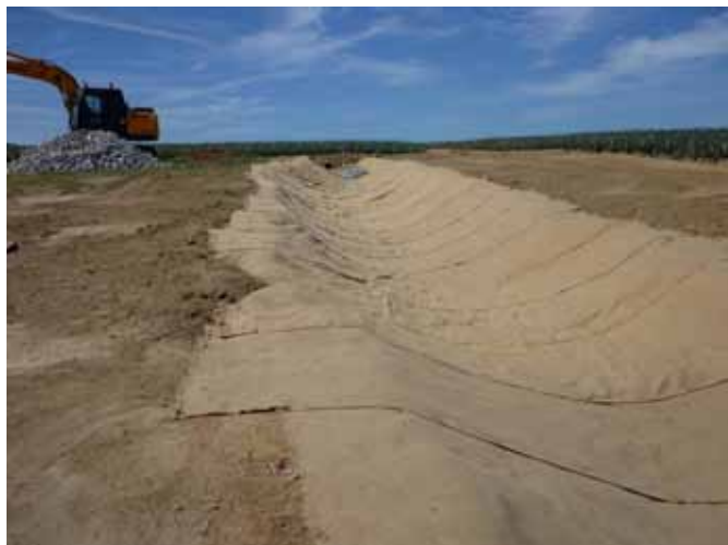
Figure 10. Drain redesign on a pineapple farm using geo-fabric as a soil surface stabiliser and later planted out with vetiver grass to aid stabilisation.
